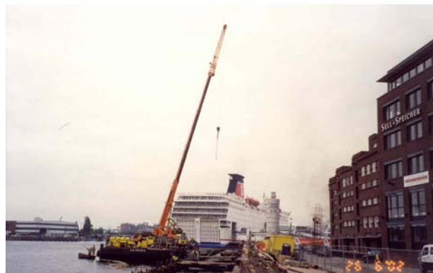
Fig. 8: Pfahlherstellung vor dem Sell-Speicher. Fig. 8: Execution of piles in front of Sell-Speicher.
